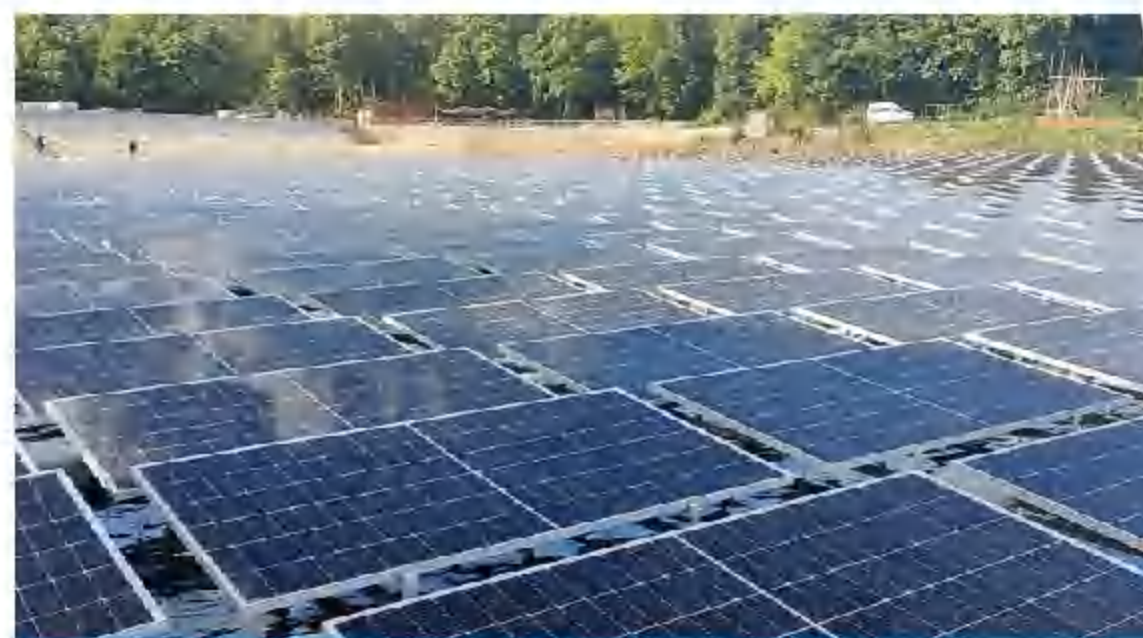
▶ Shaoxing 2MWp Surface Power Station
