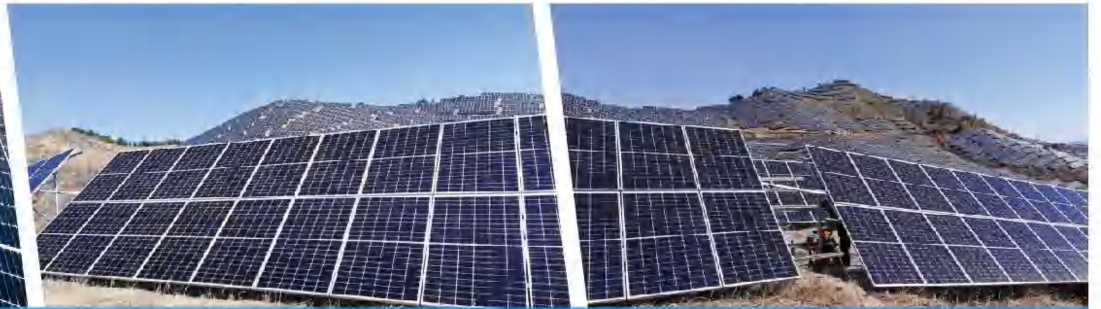
▶ Hebei Chengde Ground Power Station
