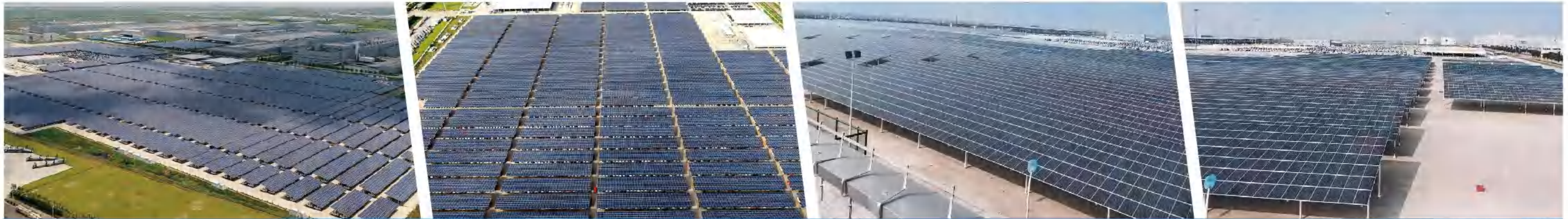
▶ Hangzhou Bay SAIC Volkswagen Plant PV Project
