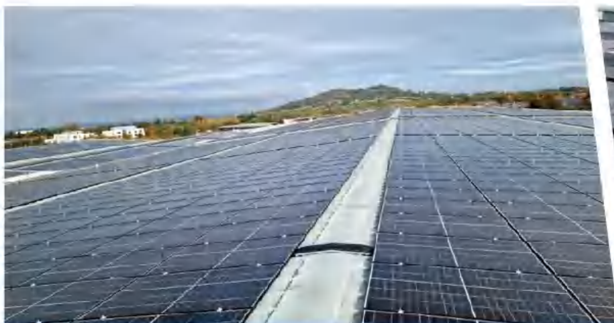
▶ 5MW project in Munich, Germany
